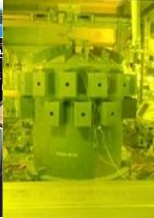
Metal Waste Furnace
